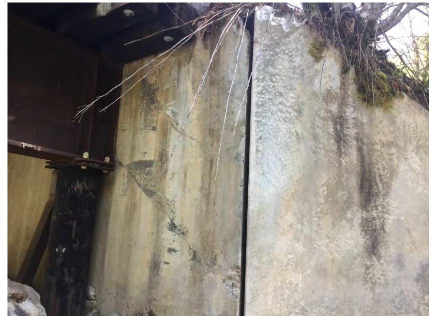
Damage noted to upstream right ballast wall
