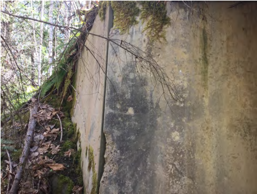
Damage noted to downstream right ballast wall
